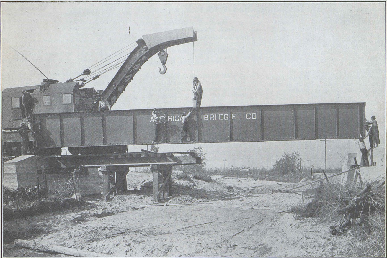
Placing one of the large steel girders spanning Eaton's Wash in connection with extension of Alhambra-San Gabriel line.
