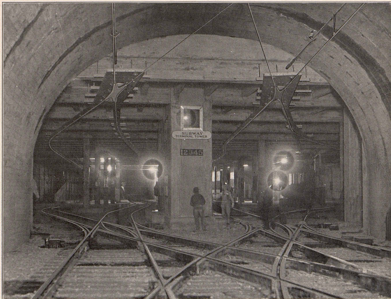
Showing overhead construction leading from subway to terminal. Note pan-switches, insulator guards and direct suspension trolley.
