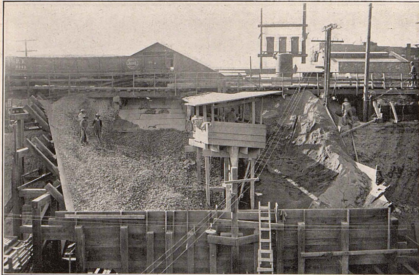
Material track and bunker, showing method of receiving and storing material employed at Figueroa Street shaft.
