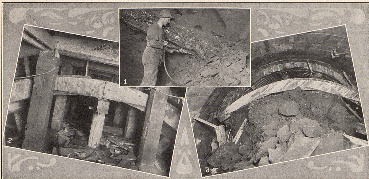
1—Workman using pneumatic air spade for removing material from tunnel drifts. 2—View showing arch segments in place prior to removal of tunnel sets. 3—Stripping forms from arch of tunnel. The remaining core will be seen in the foreground.
