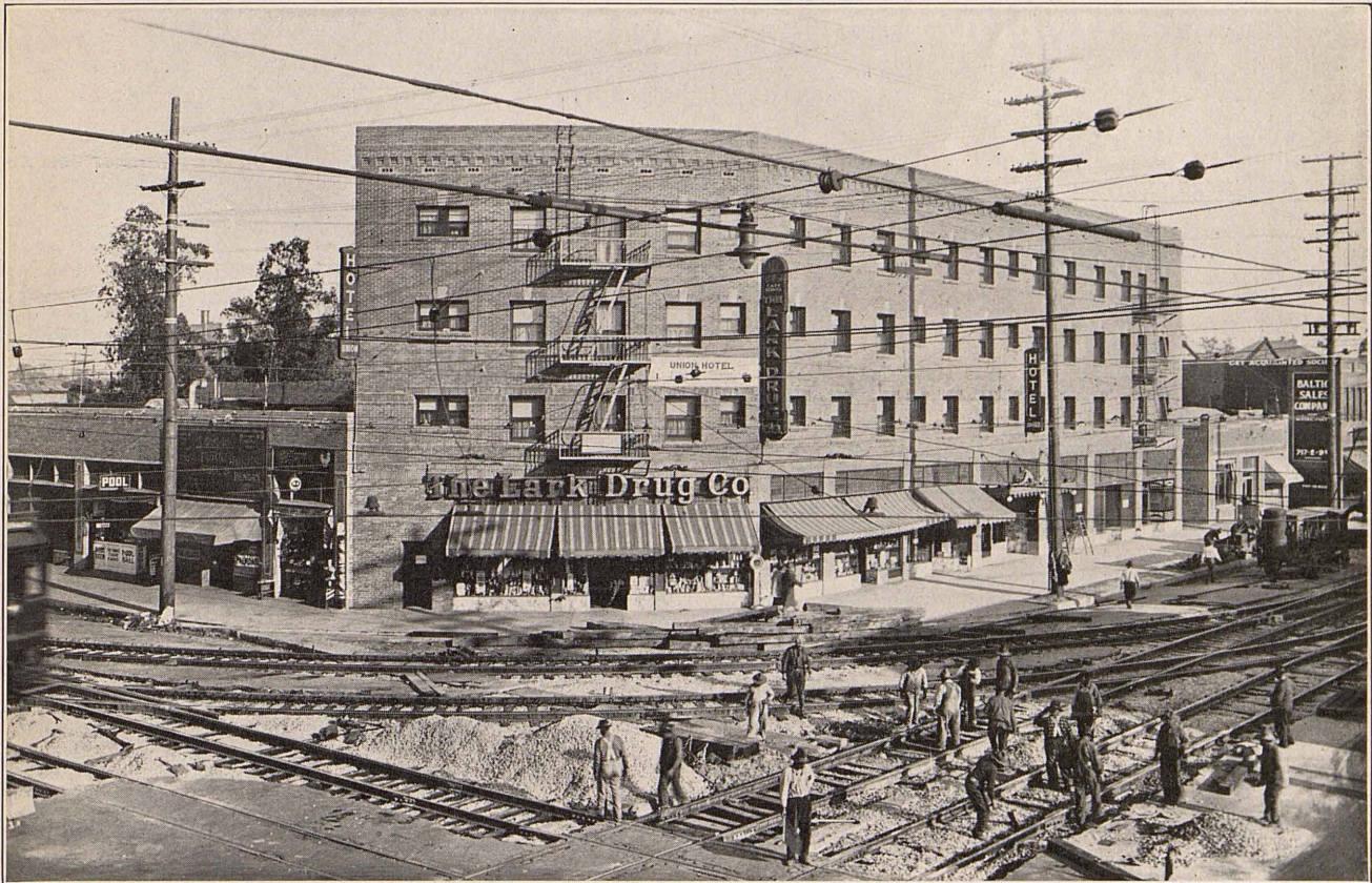
Considerably new freight traffic and speedier service will result with the servicing last month of the new double curve track layout at 9th and San Pedro Streets, shown above during progress of work.
