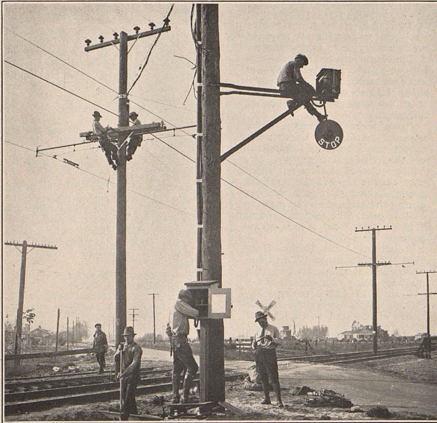
An even 500 crossing "wig wags" are now in service on P. E. lines. Photo shows Foreman Fuller and crew making an installation at West Chapman on the Santa Ana line.
