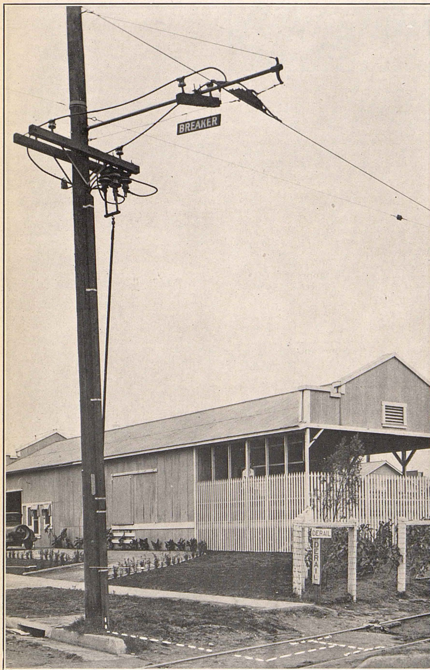
View showing combined trolley wire and track sectionalizing switch in open position.
