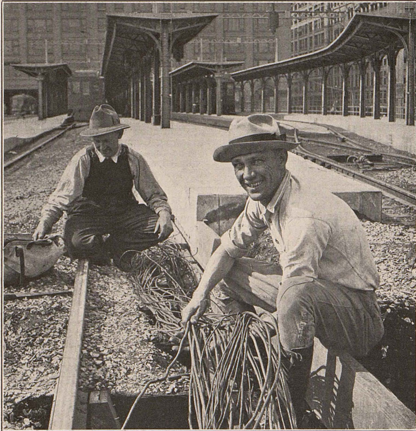
Replacing the wiring of Ma'n St. Terminal Interlocking Plant, now under way, involves the installation of some 47,000 feet of insulated wire. The heavier and better type used should withstand for twenty years.
