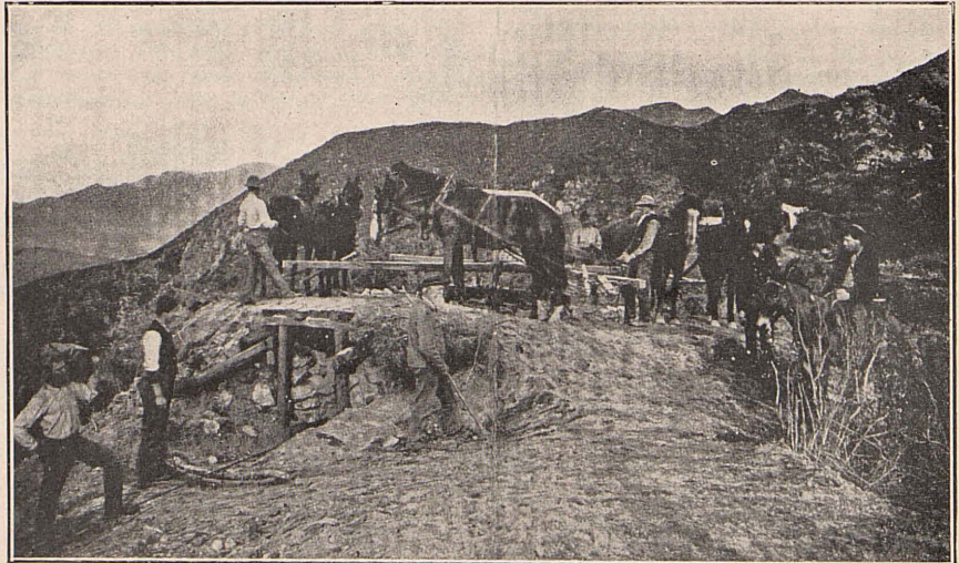
The above picture tells at a glance the construction difficulties and crude engineering equipment used in connection with the building of the Mt. Lowe incline in the early nineties. All materials and supplies were drawn to top of incline by means of the hoisting spindle shown, it requiring two hours to negotiate the grade, six horses being used as motive power.
