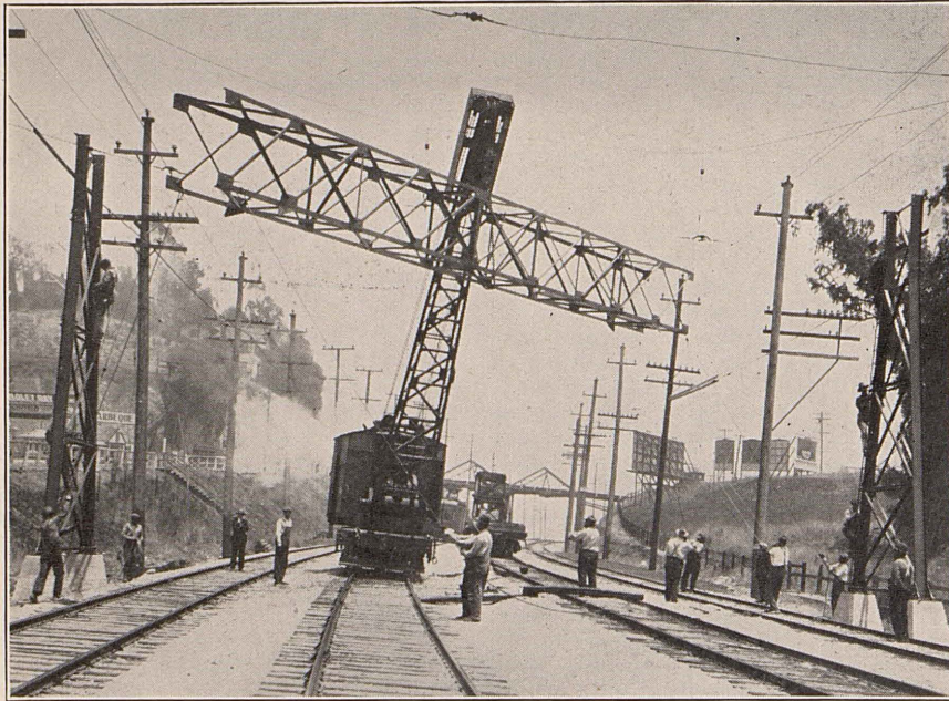
Cross spans for eight new signal bridges were last month placed in position by Company Engineering forces without major interruption to service.
