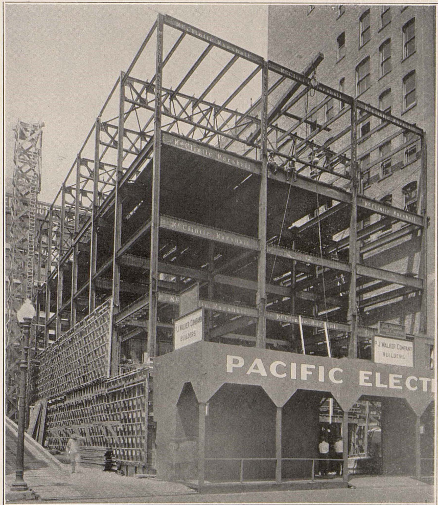
Just two months ago the cover picture on our Magazine showed Mr. Pontius participating in the time-honored ground breaking ceremony in connection with initiation of work on our new Club Building. That “it wont be long now” is evidenced in the progress picture above.
