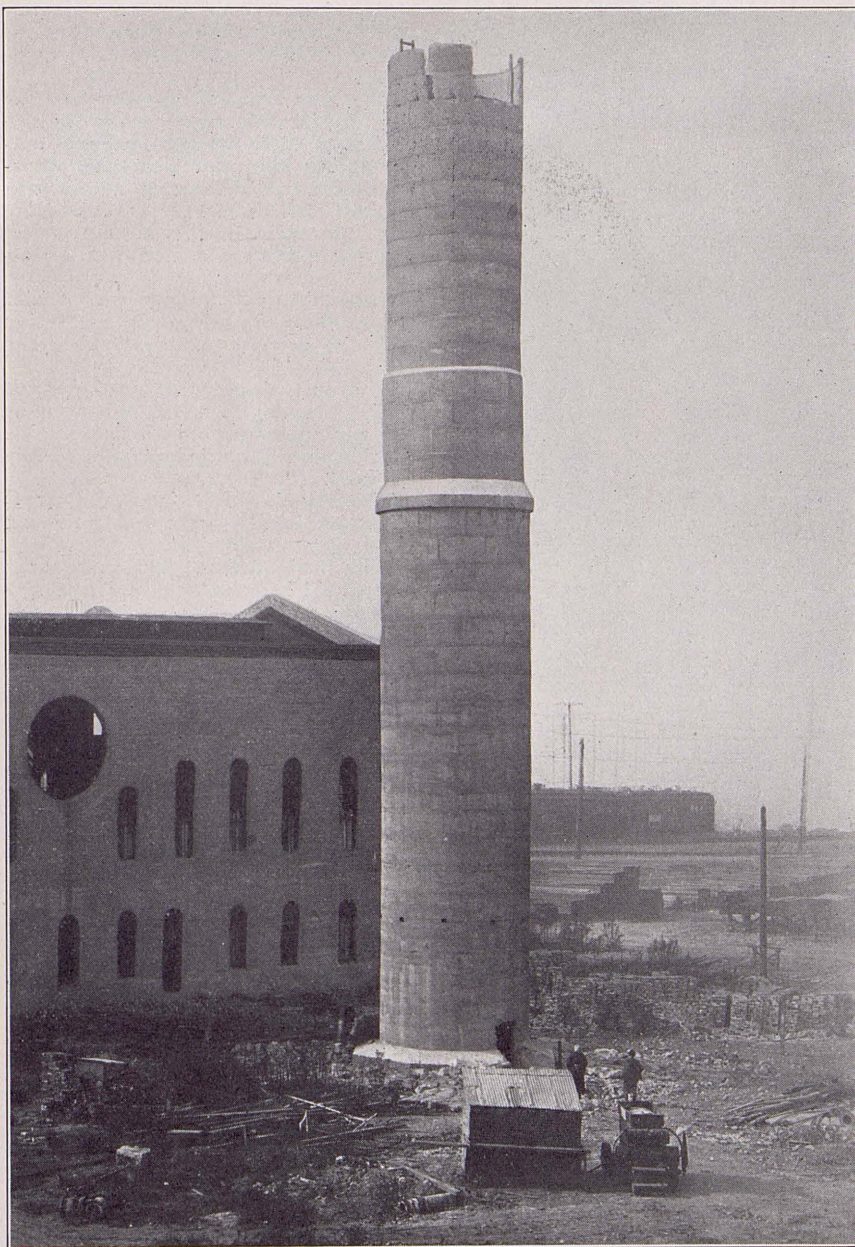
Towering 156 feet in its heyday, the concrete stack at the old Vineyard Junction steam generating plant was razed last month.
