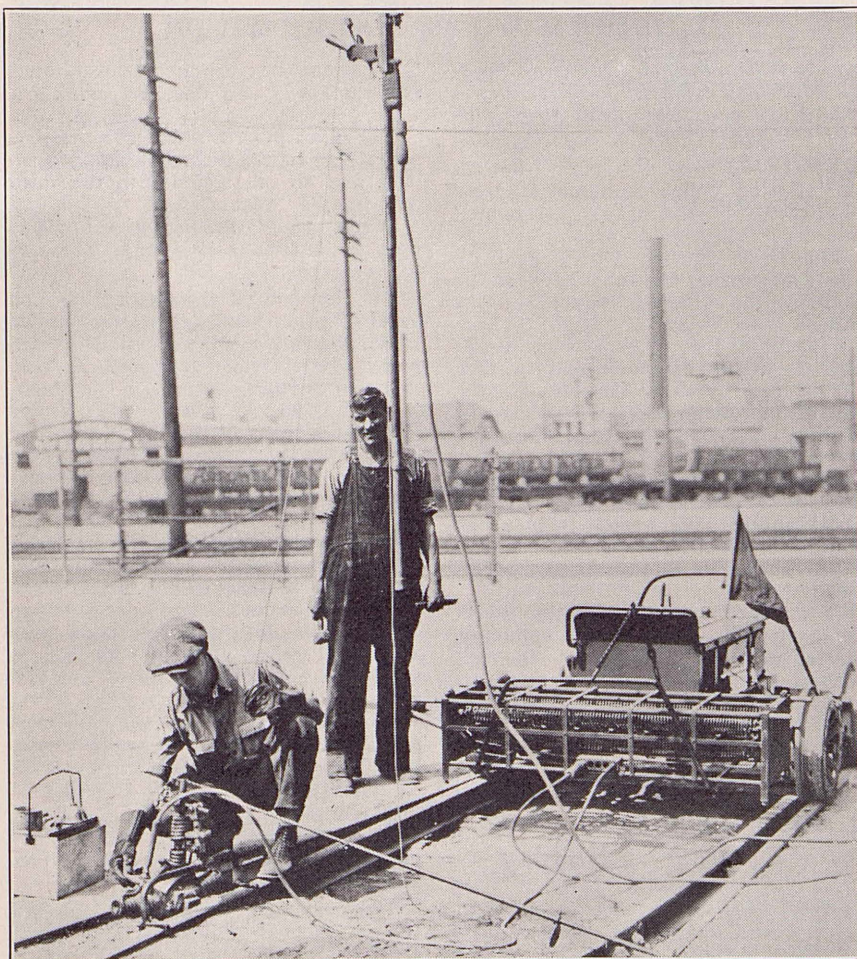
New portable bonding equipment recently put into service. One of its outstanding features is that it can be quickly lifted from tracks when train approaches. Eight of these units were purchased and their improved method will effect a large annual saving. George Prell (standing) and H. P. Bancroft are seen in the picture.
