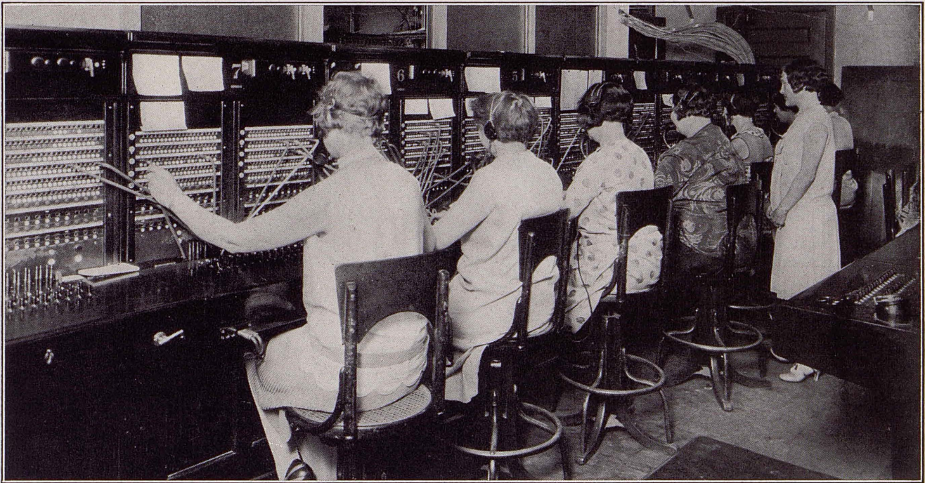
Simplifying, speeding, and otherwise improving telephone service, the Southern Pacific-Pacific Electric switchboard was consolidated last month. About $8,000 was expended upon the new layout.
