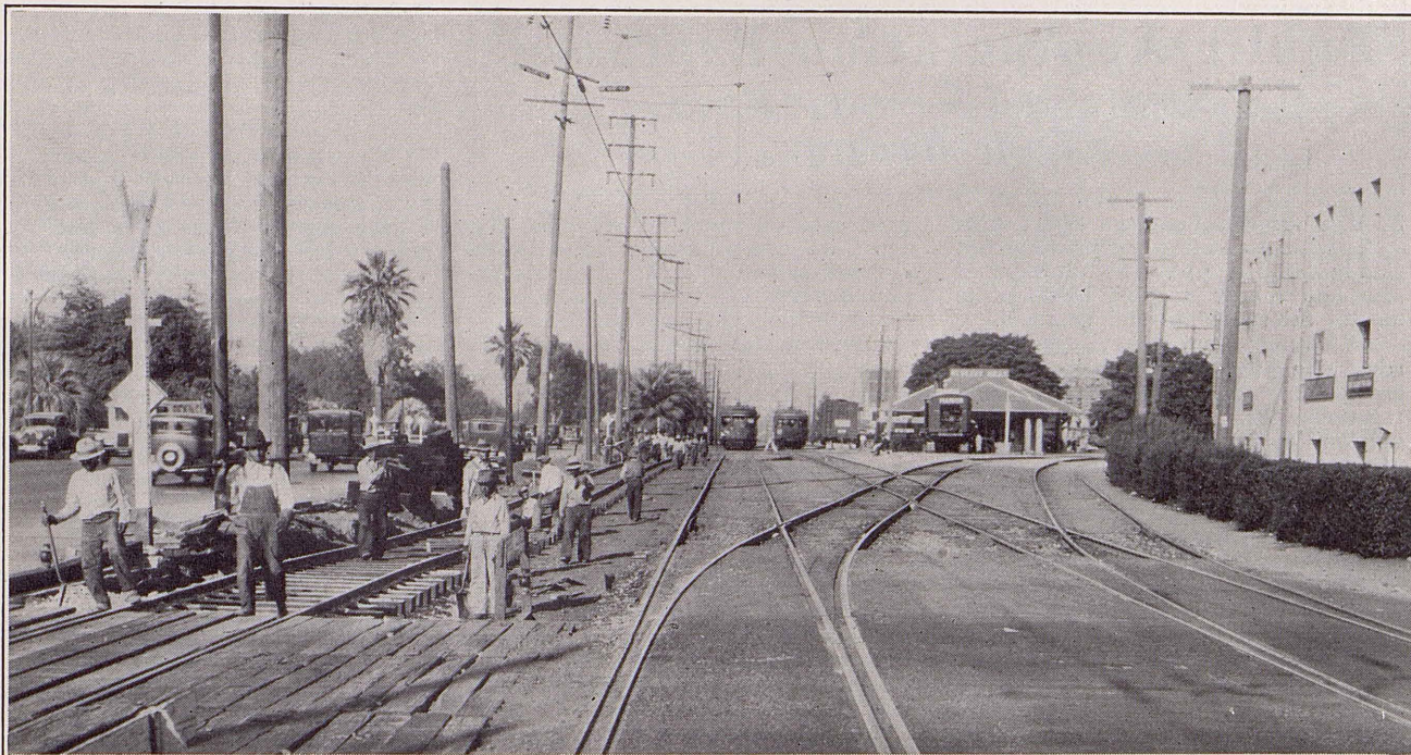
Co-operating with the City of Beverly Hills in its ambitious Civic Center program, representing an outlay of close to a million dollars, our Company is now engaged in extensive track re-location near and approaching the site which is east of the Junction between the Hollywood Boulevard and W. 16th St. lines. A beautiful new station, in harmony with architecture and design of civic buildings, is now under construction.
