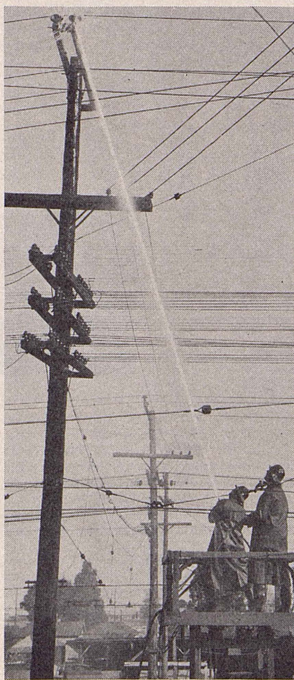
Cleaning of insulators by forced stream, enabling three men to do the work of fifty, is a new practice successfully demonstrated and adopted by our overhead line forces.
