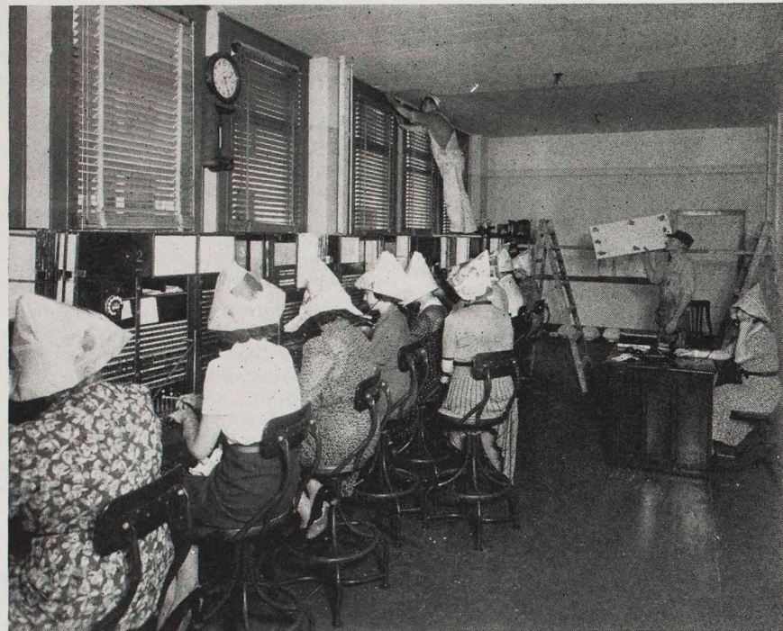
EMERGENCY UNIFORMS IN THE 'PHONE ROOM Even newspaper bonnets can't detract from the attractiveness of our Telephone Operators; but, folks, we must protect our permanents. There will be no more "wrong numbers" after the "sound-proofing" is finished.
