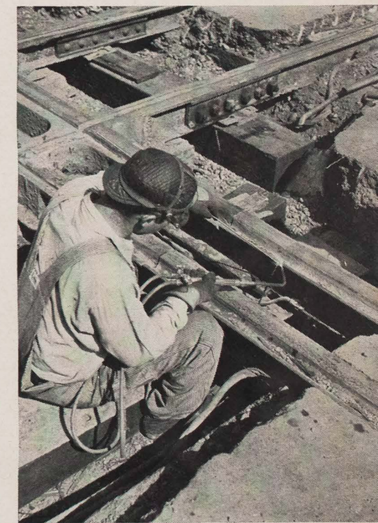
Workmen repair crossing at a busy intersection in downtown Los Angeles. Acetylene welder mends break in 128-lb. manganese steel rail.
