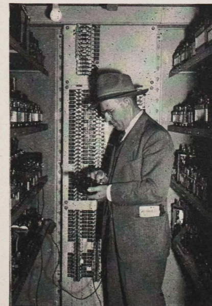
RELAY HOUSE, showing W. E. Stratman, Signal Foreman, testing relays that control signals and switches. Without these relays, the centralized traffic control system would not operate. A relay house is located at each junction and each crossing.
