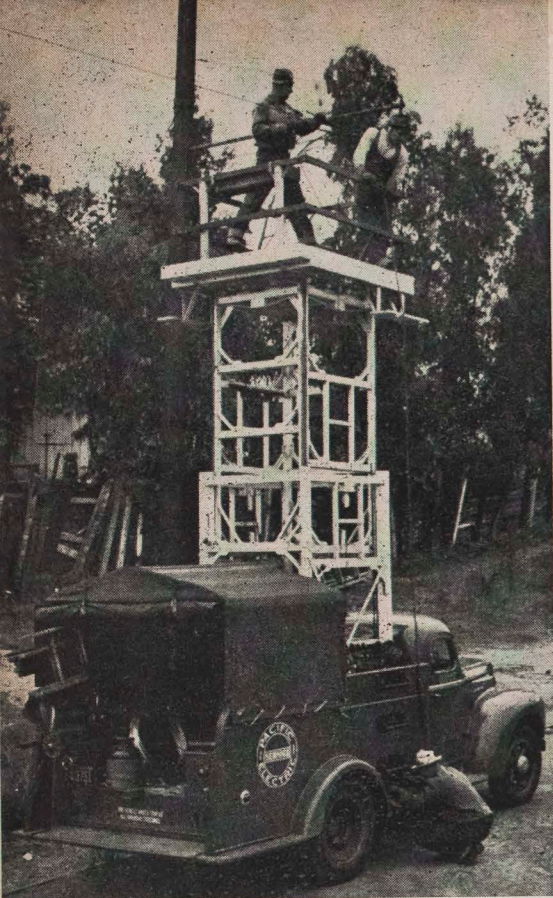
TOWER TRUCK —Splicing a trolley at Macy Street are Lineman F. B. Hooper (left) and Crew Foreman R. E. Thompson. Driver C. H. Poole is looking for a trolley dog.
