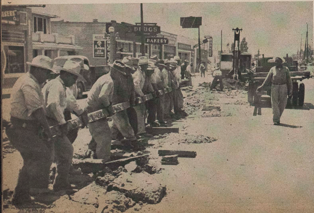
REMOVING 60-POUND RAIL on Highland (Arrowhead line) San Bernardino, and excavating to relay roadbed with 128-lb. grooved girder rail taken from abandoned San Bernardino-Colton local line. The excavator is the tall machine in the background. Part of Extra Gang No. 9 is carrying the rail.
