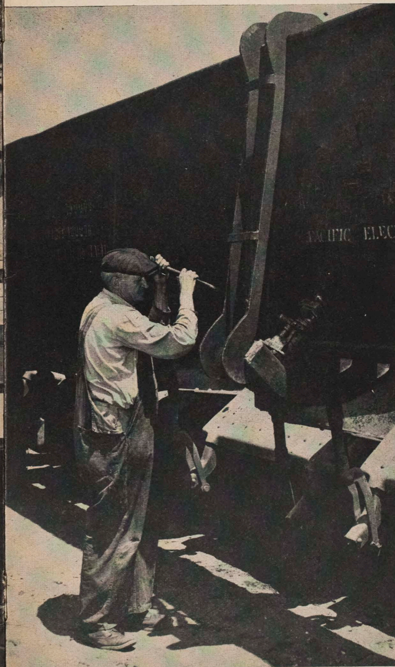
PUSHING IN THE SIDE OF A STEEL GONDOLA with a hydraulic jack is Car Repairer John Prestegaard at Butte Street. By the old method, the car had to be chained down and jacks braced, and it would take two men all day to even up the sides of one car. Now, with the straightener developed by Butte Street shop forces, two men can do the job in two hours.
