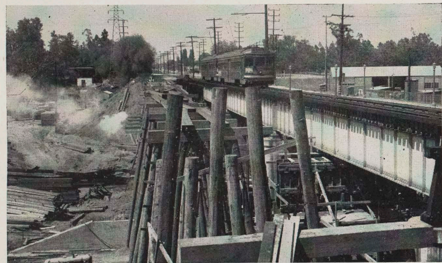
RAIL TRESTLE over Los Angeles River at Vineland Ave., North Hollywood, will soon be torn down and rebuilt by U. S. Army Engineers as small part of big flood control project. Pilings in unfinished structure in picture are for temporary shoofly to be used by Valley trains pending rebuilding of trestle over which train is moving.
