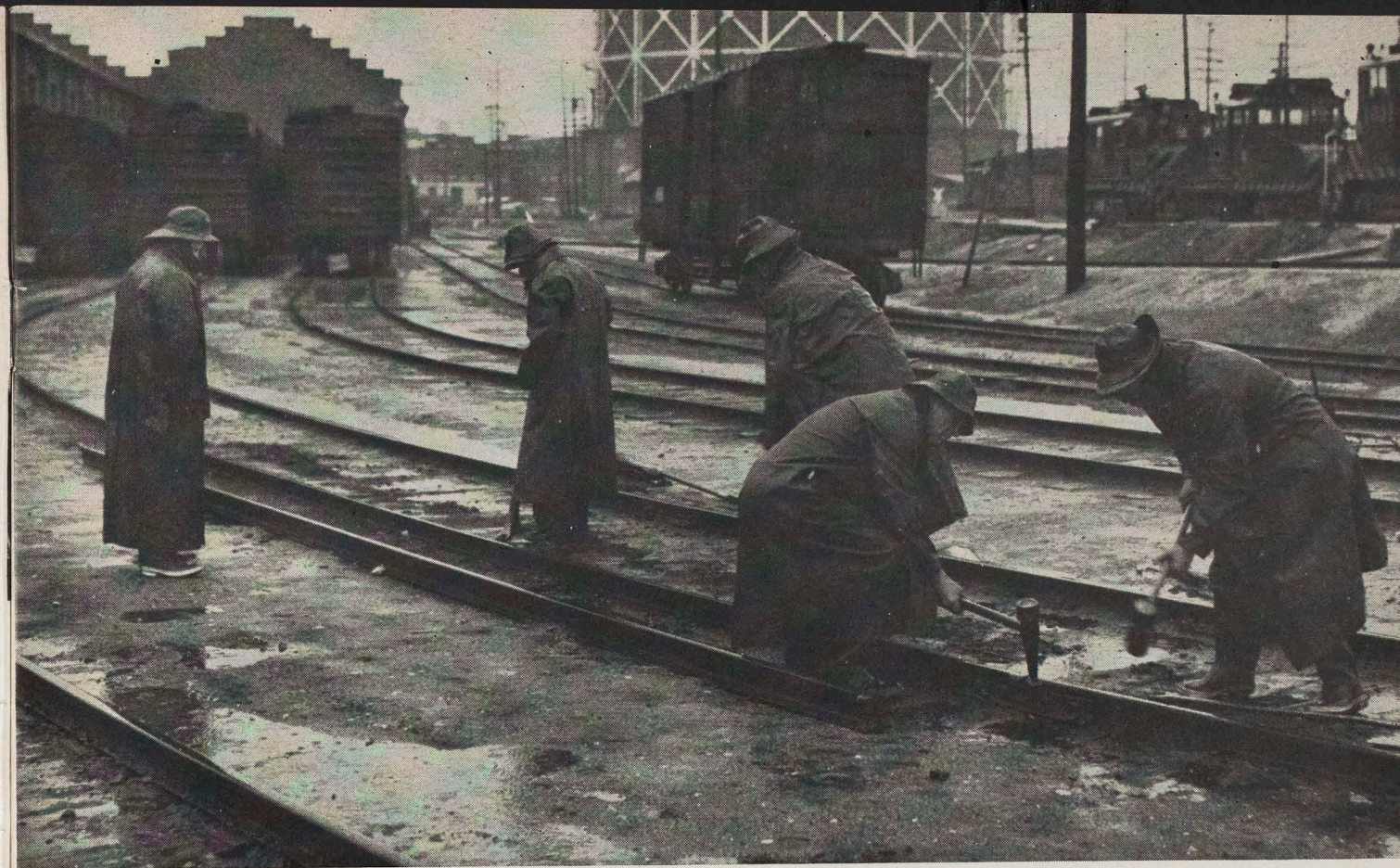
RAIN NO HINDRANCE —In raincoats, boots, and rain hats, Section 15 at Eighth St. Yard prepares to replace a rail in wet weather. Foreman Jesus Fonseca is at left. When it's raining, gangs are careful in handling slippery tools, and must watch for slippery footing.
