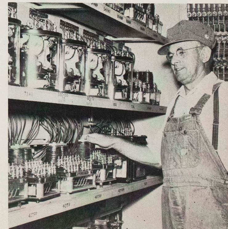
INSPECTS RELAYS —Signalman John Huber has been maintaining the interlocking plant at Watts since 1925. These are the intricate relays without which the plant couldn't work.
