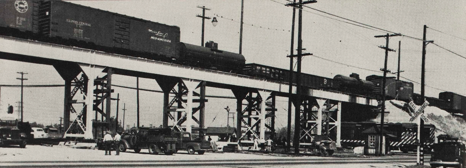
↑ TRAINS KEPT MOVING even though the PE bridge over the Santa Fe tracks just west of San Bernardino was in process of being raised. While the train pictured was crossing, bridge had been raised 9 inches, but was not allowed to rest on jacks.
