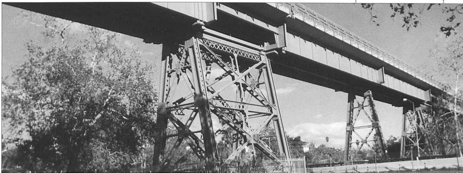
The Arroyo Seco Bridge located in the Highland Park/South Pasadena area has been rehabilitated thanks to funding from the MTA. The bridge was first completed in 1894. The structure was rebuilt in 1913 and again in 1923. Restored in keeping with its original style, the bridge will become part of the Metro Blue Line to Pasadena.
