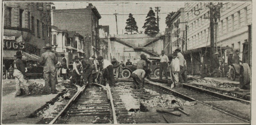
Picture shows installation of new special work at Temple Street and North Broadway, this being the first part of the job.
