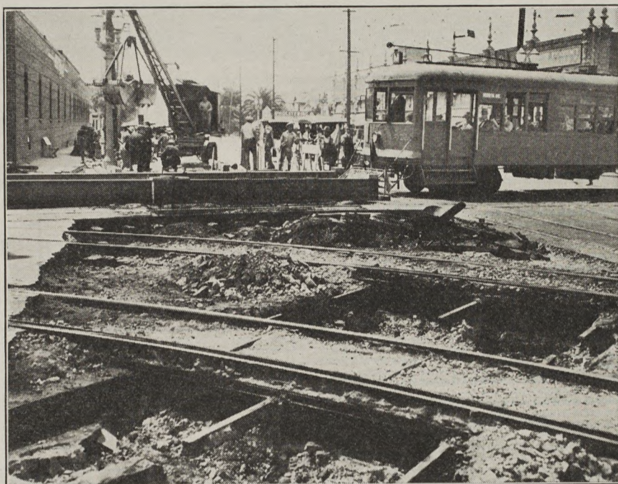
First step in work begun last week by the Ways and Structures Department. Bridge work is being installed for the support of the car tracks over the excavation of the West Jefferson Storm Drain.
