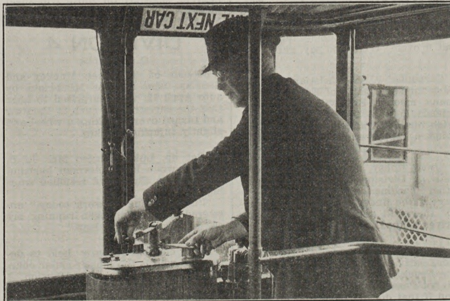
Picture shows W. R. Cavett, inspector of operating equipment, applying remedy to frozen controller, which might have saved 32 minutes' delay at the end of a line.
