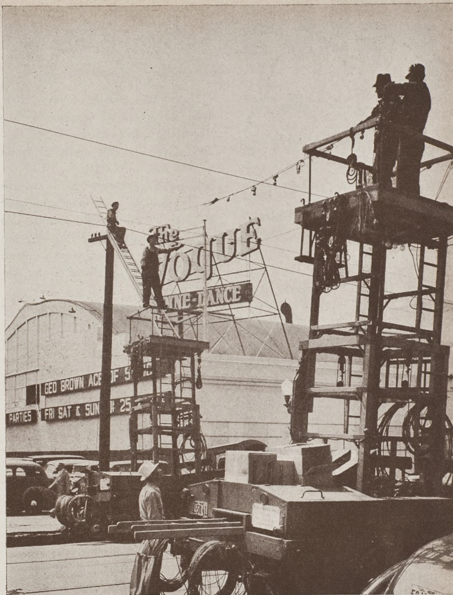
Two of our Tower Trucks removing overhead lights which have been in use since 1907.
