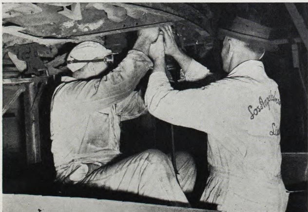
● Fred Anderson, group leader, aids Frank Young beneath the street car as they make preparation to put on lifeguards.
