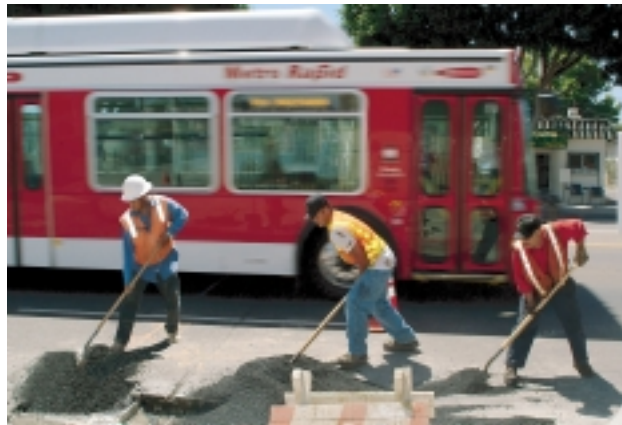
Los Angeles Department of Transportation subcontractors install Metro Rapid signal priority sensors at Florence Avenue and Gramercy Place.
