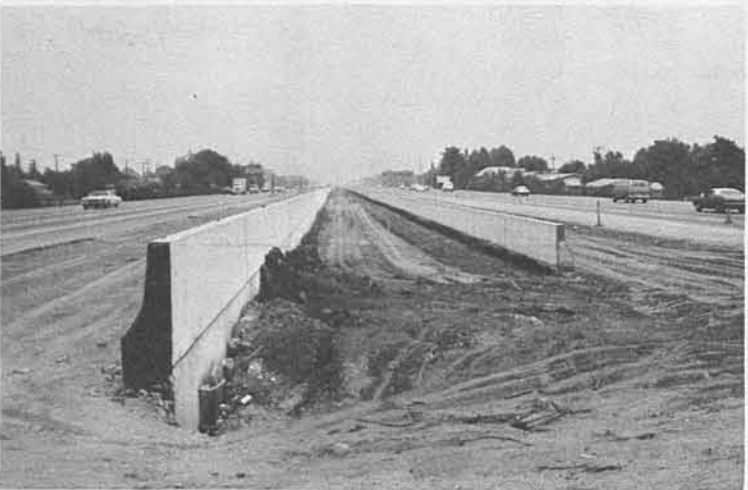
Sub-grade work on this portion of the Busway has been completed. Soon a section of Southern Pacific Railroad tracks will be laid between the concrete barriers with busway lanes on the outside of the barriers.
