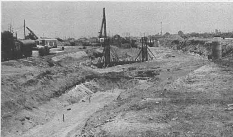
Construction of an overpass for Southern Pacific Railroad tracks is underway west of the El Monte Busway Station. Busway buses will travel under the tracks entering and leaving the Station.
