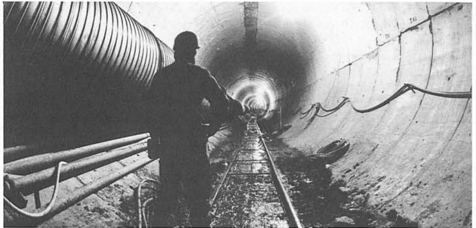
Digging the tunnels is a lonely job and it goes on around the clock
