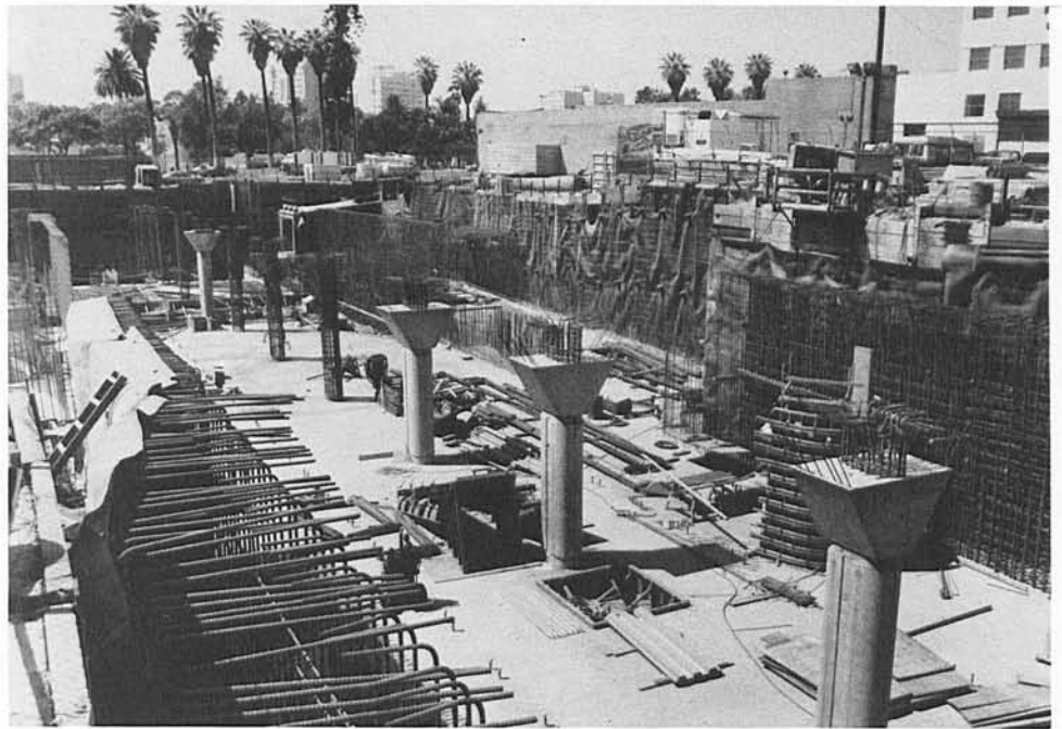
CONCRETE SENTRIES STAND GUARD NEAR MacARTHUR PARK—75-foot tall concrete supports keep a stark vigil over the Westlake-MacArthur Park Station site at Wilshire and Alvarado, the western terminus of the first 4.4-mile segment of RTD's Metro Rail subway project. Excavation of the station is nearly complete, and will be followed by "Stage II" work which includes installation of elevators and escalators, tile work and other esthetic touches. The $1.25 billion project has been under construction for almost three years and is expected to open for service in September, 1993.
