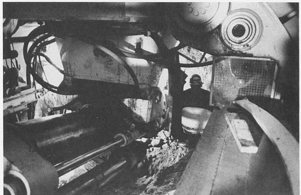
DIGGING FOR A LIVING — The eerie, cylindrical world of tunnel diggers greets these workers each day on RTD's Red Line project. Once inside this ever-lengthening tunnel fragment (top photo) near the future Union Station subway terminal, it is impossible to tell the difference between night and day. In the bottom photo, a lone tunnel digger operator is dwarfed by the huge hydraulic hindsection of the machinery that is creating the Red Line's tunnels.
