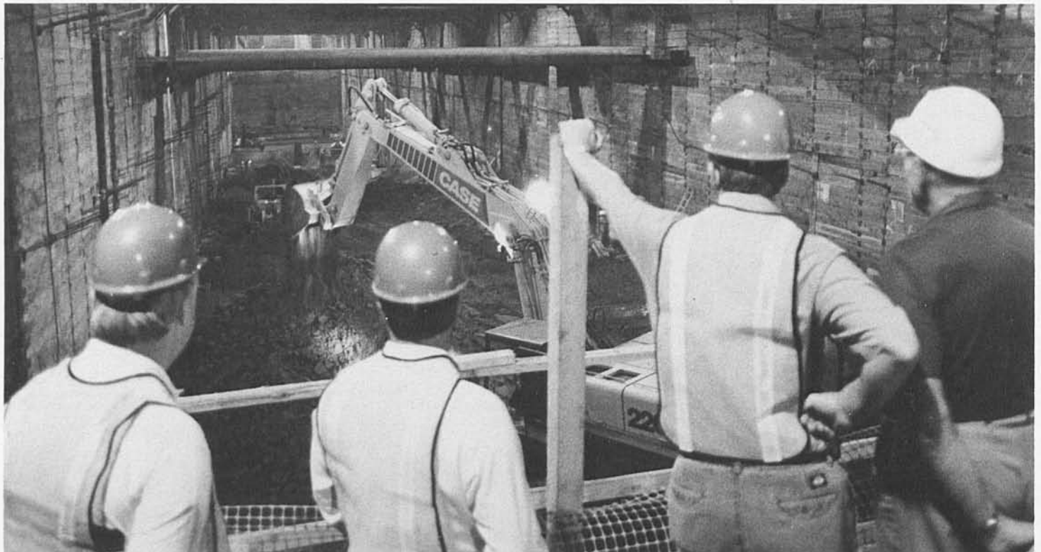
The future Civic Center Red Line station at First and Hill streets will be 55 feet wide and 570 feet long.
