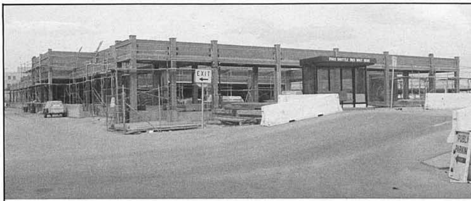
A new baggage handling facility is part of the Metro Red Line interface at the Union Station in downtown Los Angeles.
