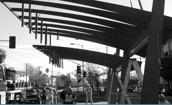
Workers guide the overhead canopy into place at the Metro Orange Line Laurel Canyon Station at Laurel Canyon and Chandler Boulevard in North Hollywood.
