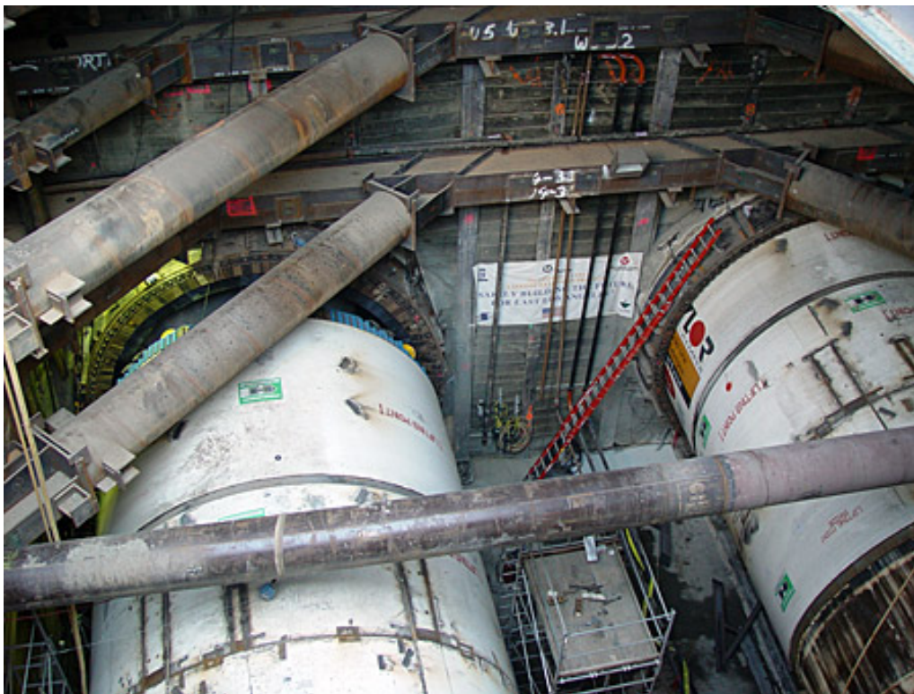
Gold Line Eastside Extension Project – boring a 21-foot, 4-inch-wide tunnel under East Los Angeles
