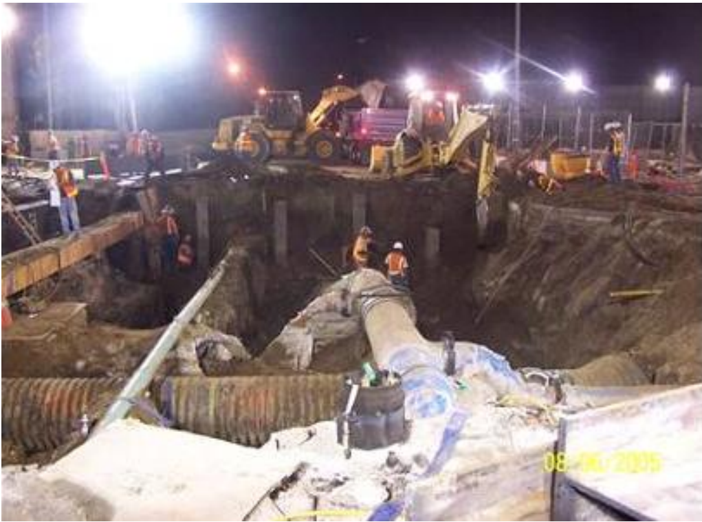
Gold Line Eastside Extension – excavation for south row of piles at Soto Station
