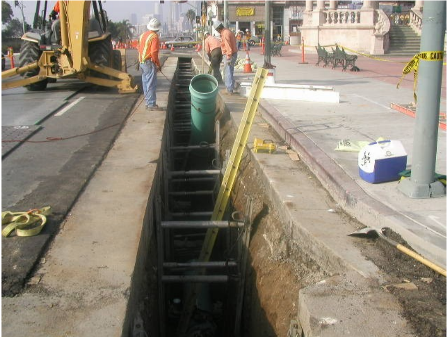
Gold Line Eastside Extension -- Placement of 18" storm drainage line at 1st and Boyle Avenue
