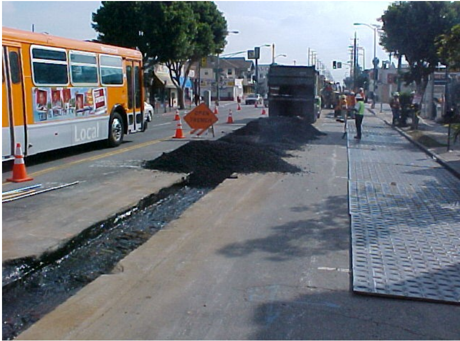
Gold Line Eastside Extension -- Repair of 1st Street after relocation of 12" water line
