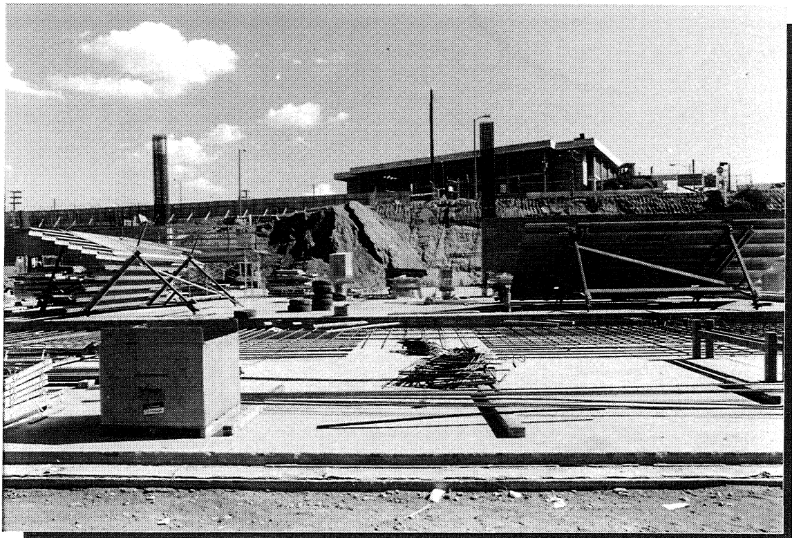
PUBLIC TRANSIT PARKING – LOOKING EAST SLAB ON GRADE: MUD SLAB, WATERPROOFING, PROTECTION SLAB, PARKING SLAB
