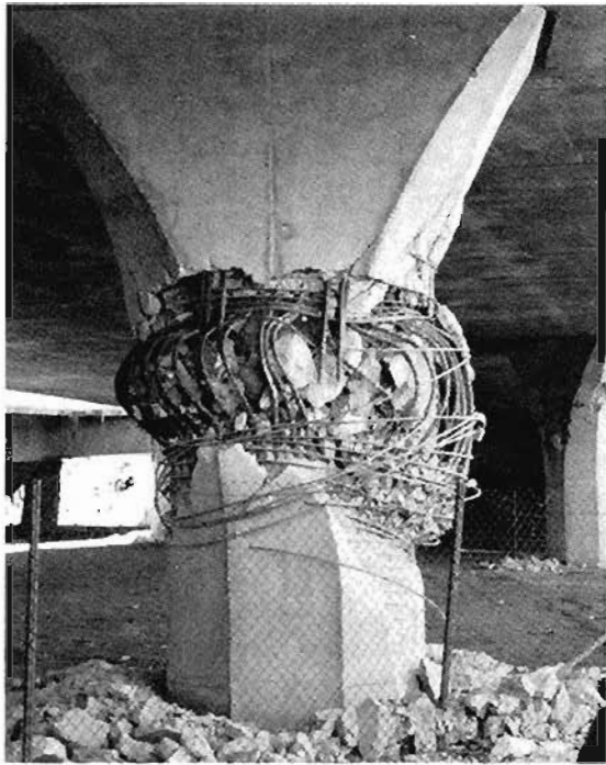
Figure 4-7. SR-118 Mission & Gothic Undercrossing, Northridge earthquake. (photo: F Seible)
