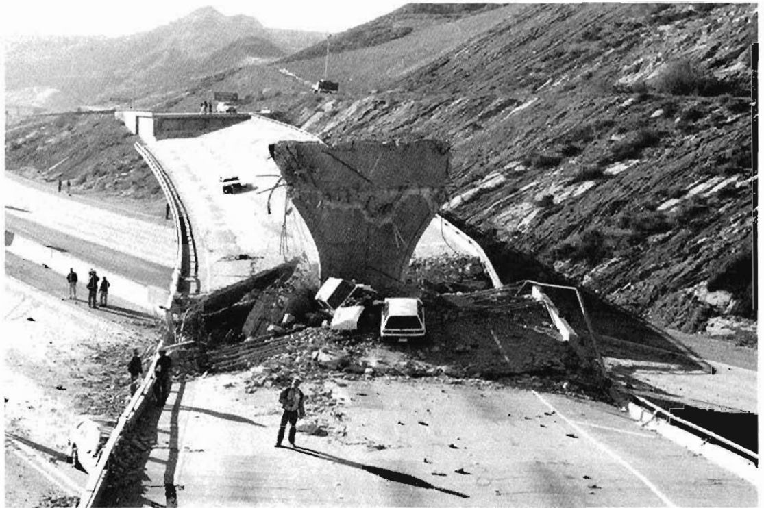
Figure 4-5. SR-14/I-5 South Connector Overhead, Northridge earthquake. (photo: F. Seible)
