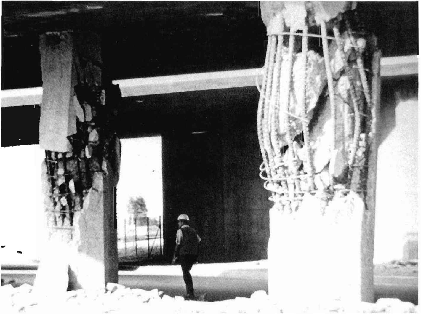
Figure C-3. Columns of the San Fernando Road Overhead suffered heavy damage during the San Fernando earthquake. Note the similarity to the performance of the I-118 Mission and Gothic undercrossing in the Northridge earthquake, Figure 4-6. (photo: National Earthquake Engineering Information Service archive)
