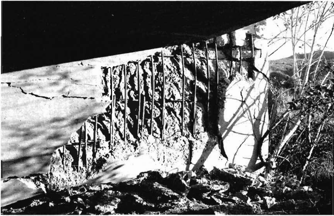
Figure 3-9. Abutment joint damage in the separation structures at the Antelope Valley I-5/SR-14 Interchange (photo: F. Seible)
