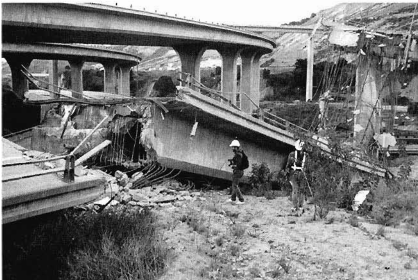
Figure 4-4. SR-14/I-5 North Connector Overcrossing, Northridge earthquake. (photo: F. Seible)
