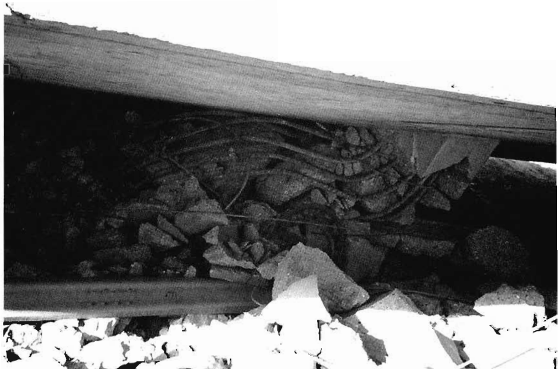
Figure 4-6. Short column failure SR-14/I-5 South Connector Overhead, Northridge earthquake. (photo F. Seible)
