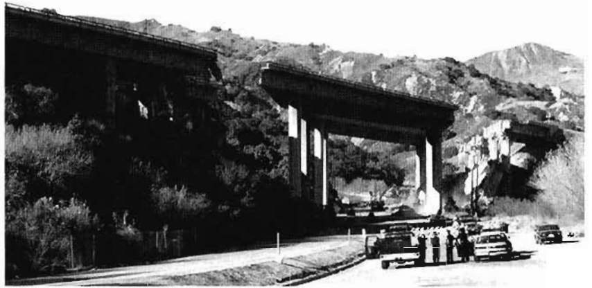
Figure 3-11. The highly skewed geometry and short expansion joint seat width of the still-standing center frame of the I-5 Gavin Canyon bridge. (photo: F. Seible)
