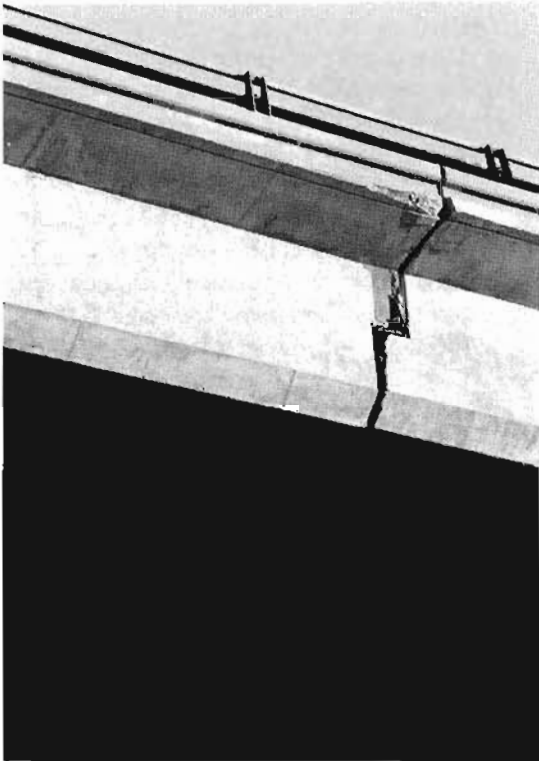
Figure 3-10. Expansion joint damage in the separation structures at the Antelope Valley I-5/SR-14 Interchange (photo: F. Seible)
