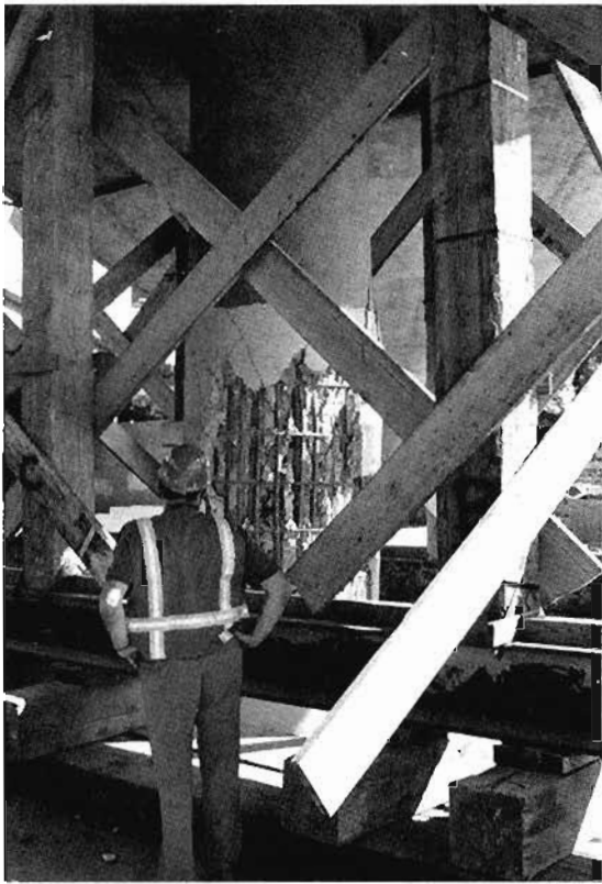
Figure 3-4. Steeply inclined shear cracks and cover spalling in one bent at Fairfax & Washington on I-10 (photo: F. Seible)
