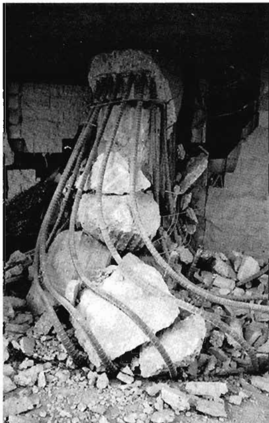
Figure 4-3. Brittle column failure at I-10, La Cienega and Venice. Northridge earthquake. (photo: F. Seible)
