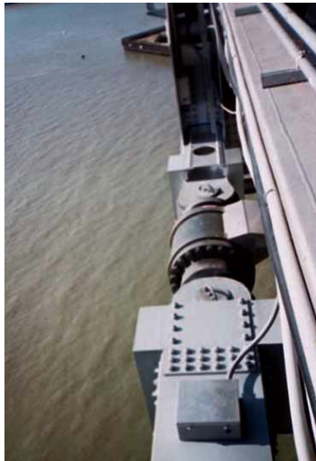
Figure 9-14. Shock transmission unit installed, Carquinez Strait Bridge retrofit.
