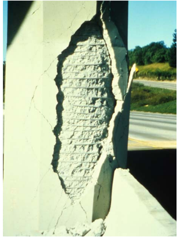
Figure 7-23. Excellent column performance on SR-118 in the 1989 Northridge earthquake.
