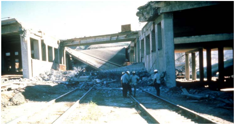
Figure 7-1. Spans slipped off narrow support seats in the 1971 San Fernando earthquake.
