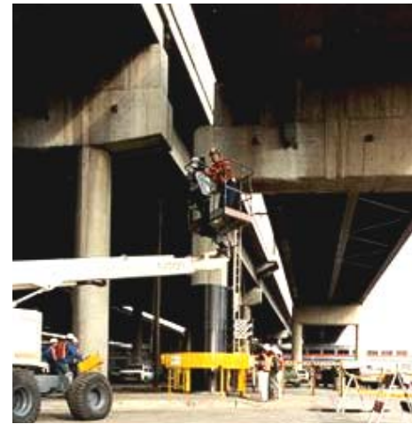
Figure 8-2. Carbon fiber jacketing of two-column bridge bent on the I-10, Santa Monica Viaduct.
