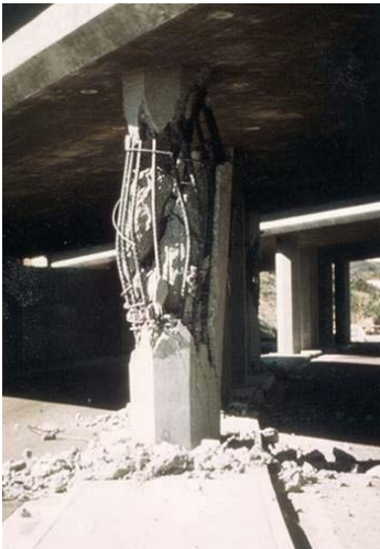
Figure 9-6. Shear failures of short columns in the 1971 San Fernando earthquake.
