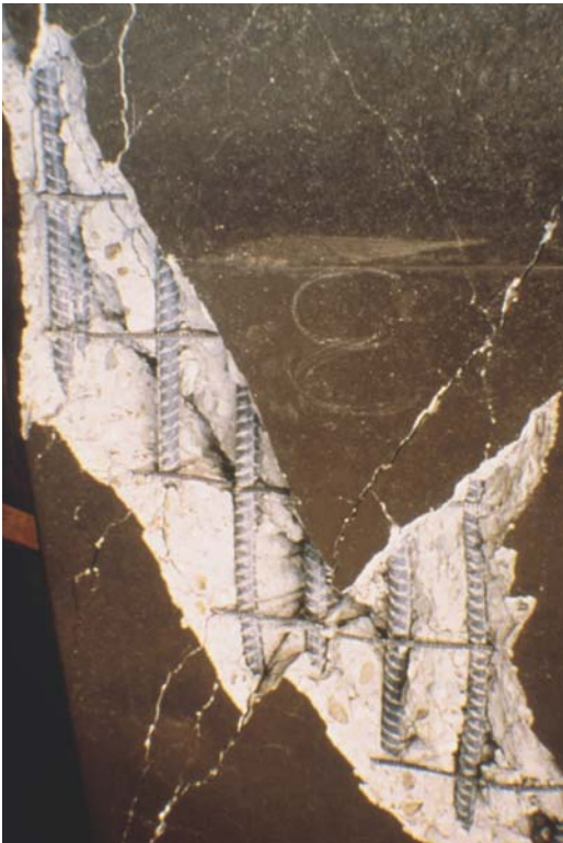
Figure 7-6. Column shear failure in the 1987 Whittier Narrows earthquake.
