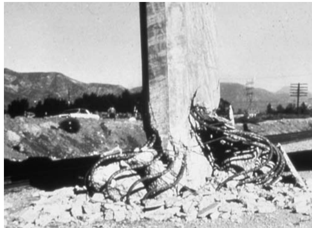
Figure 7-4. Single-column shear failure.
