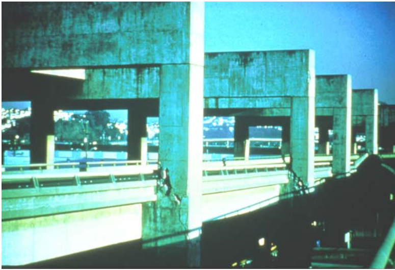
Figure 7-16. Severe column damage to the Southern Freeway Viaduct, San Francisco, in the Loma Prieta earthquake.
