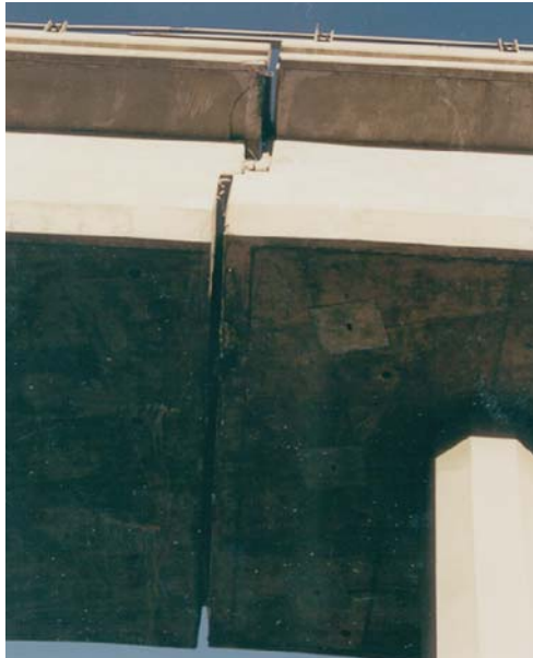
Figure 9-1. Seat width problems in pre-1971 bridge construction.
