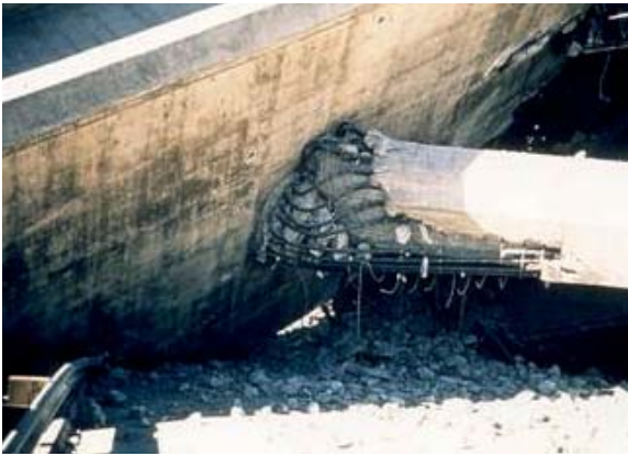
Figure 9-4. Flexural confinement problems.
