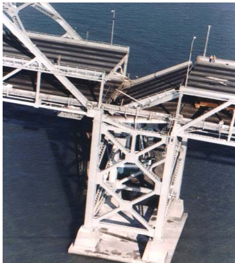
Figure 4-2. Collapse of one span of the eastern section of the San Francisco-Oakland Bay Bridge during the 1989 Loma Prieta earthquake.
