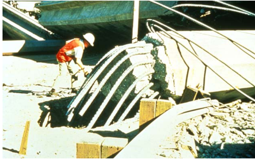
Figure 7-3. Pullout of column reinforcing steel.
