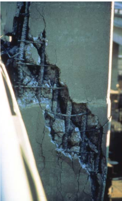
Figure 7-17. Close-up of column damage in Figure 7-16.
