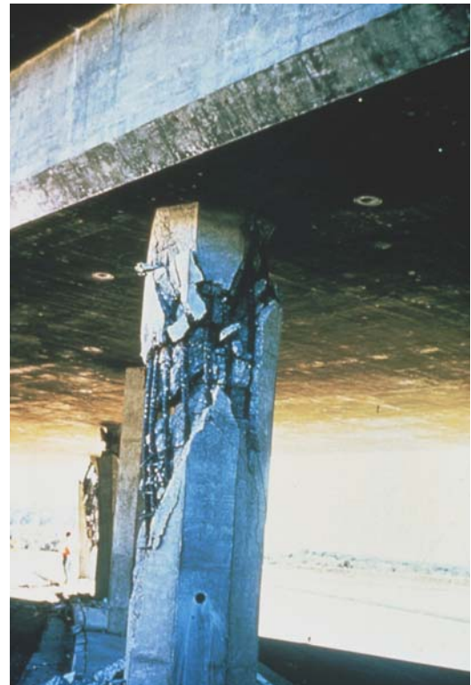
Figure 7-5. Multiple column shear failure.
