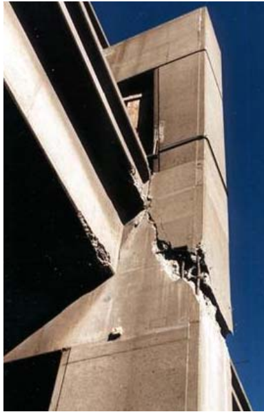
Figure 9-9. Joint failures, I-880 Cypress Street Viaduct, Oakland, in the 1989 Loma Prieta earthquake.
