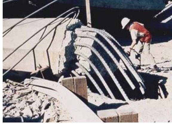
Figure 9-5. Reinforcement development problems.
