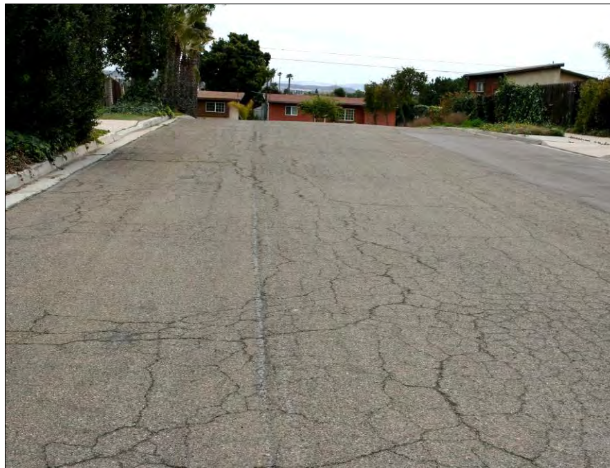
Figure 3.6 PCI = 40 (Poor Condition)
