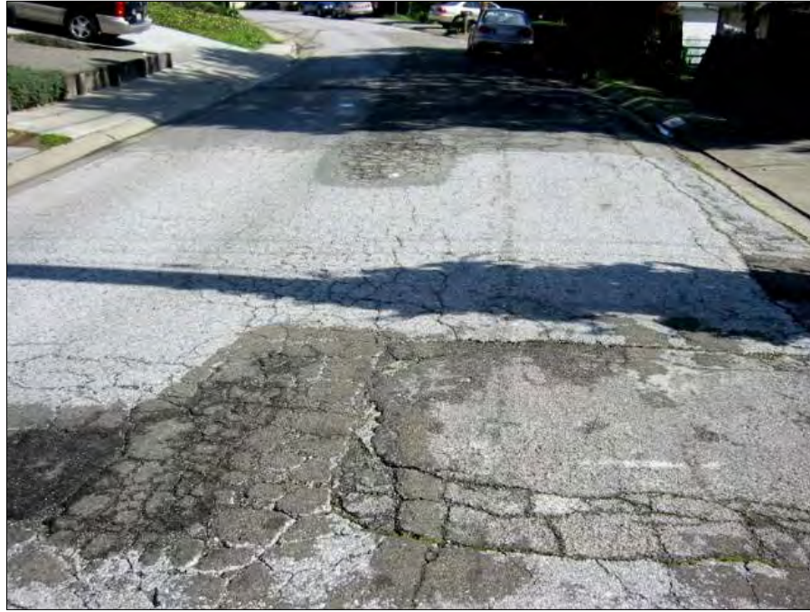
Figure 3.7 PCI <10 (Failed Condition)
