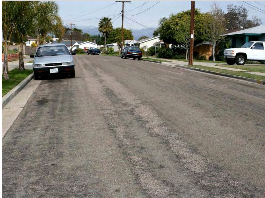
Figure 3.5 PCI = 68 ("At Risk")
