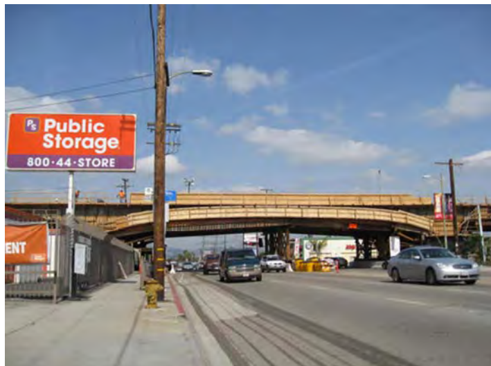
Mid-City Exposition Light Rail line construction at La Cienega Blvd and Jefferson Blvd.
