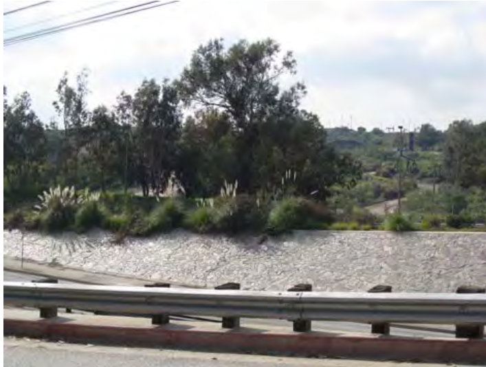
Embankment at Kenneth Hahn State Recreation area paved with flagstone & high-quality landscaping.
