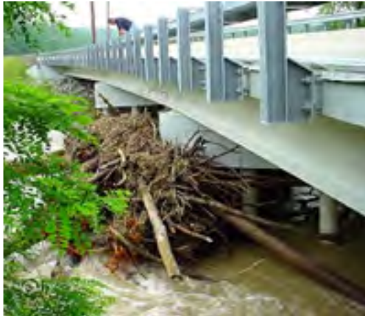
NCHRP Report 653 examines the effects of debris on bridge scour. At this bridge, a fully formed mass of debris creates significant scour potential.
