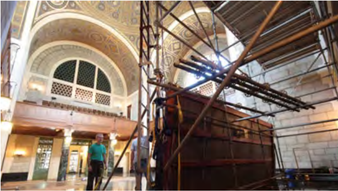
While the National Academies building on Constitution Avenue is being renovated, some TRB staff have relocated from the Keck Center to accommodate personnel from the headquarters building. (Photo: Tamara Luzeckyj, Olin Conservation, Inc.)
