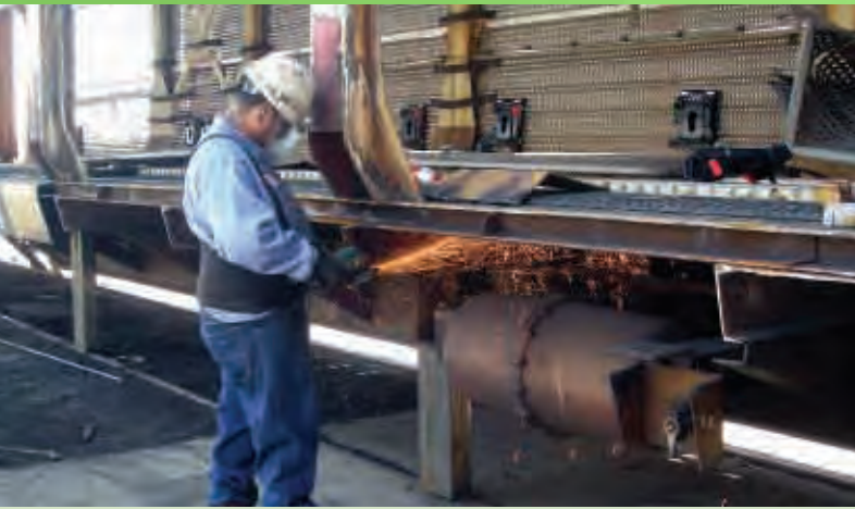
A Greenbrier employee at their Tucson, AZ facility performs a repair on a freight railcar.
