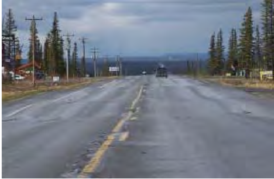
Typical permafrost damage on the Glenn Highway near Glennallen, Alaska.
