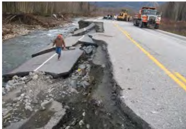
Damage on the Richardson Highway after unexpectedly high flood surges from the 2006 South Central Alaska storm.
