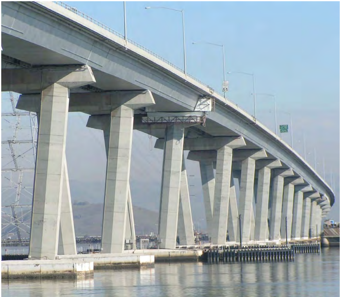
Figure 4-1. The Dumbarton Bridge, on State Route 84 between San Mateo and Alameda Counties, is to be retrofitted to improve its seismic performance following a peer reviewed assessment by BATA and Caltrans.
