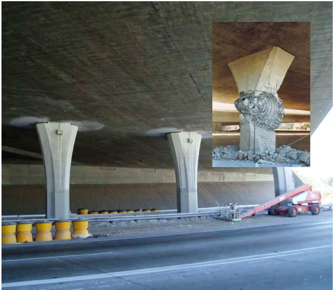
Figure 3-1. Before and after the 1994 Northridge Earthquake. Changes in design standards and details for flared columns were developed and implemented by decoupling the flares to increase the column height between plastic hinges.
