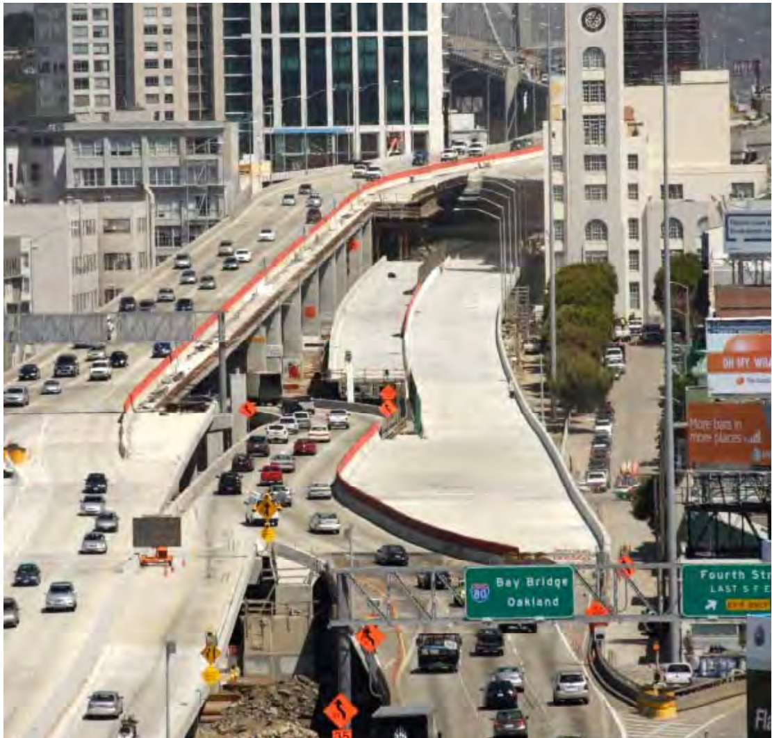
Figure 1-1. Traffic management and safety during the seismic retrofit and reconstruction of the West Approach to the Bay Bridge that required un-interrupted traffic operations for the ~ 280,000 daily Bay Bridge crossings.
