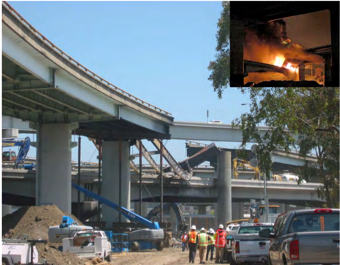
Figure 7-1. A section of the eastbound I-80 to I-580 MacArthur Maze connector collapsed following a tanker fire on the roadway below. The lower deck was reopened in eight days and the upper deck was rebuilt and reopened less than a month following the incident. [Fire Photo from Associated Press]
