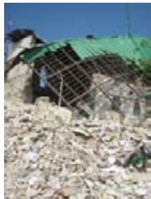
Haiti Earthquake: Ministry of Public Works
