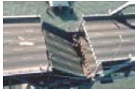
Loma Prieta damage to Bay Bridge, Oakland, CA
