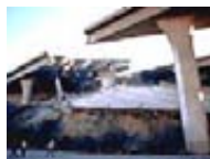
Highway vulnerability to Northridge Earthquake
