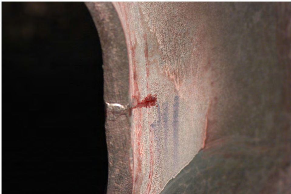
Figure 51 Fatigue cracking from seam weld in the hand hole frame of specimen VII-4
