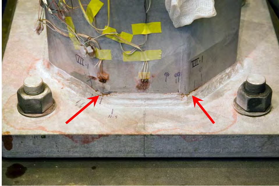
Figure 54 Fatigue cracking from toe of pole-to-transverse plate weld in pole of specimen Type VII
