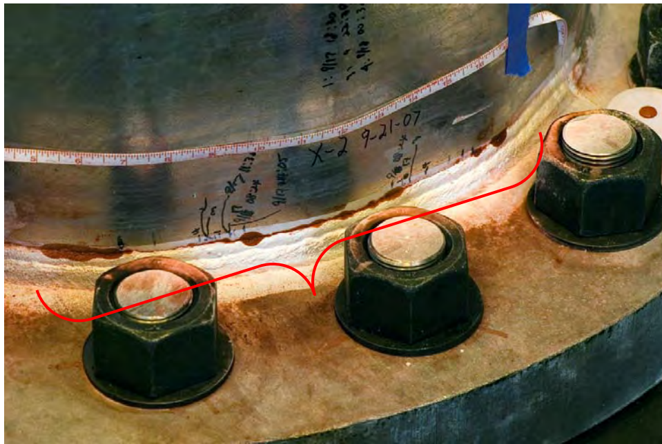
Figure 57 Fatigue cracking at pole-to-base plate fillet weld toe in high-level luminaire structure specimens
