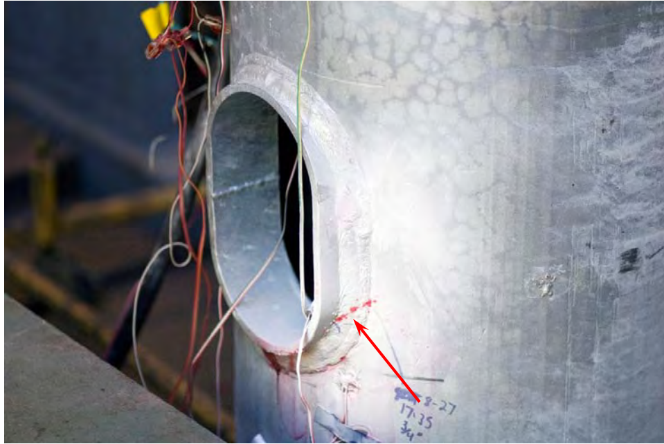
Figure 39 Fatigue crack from un-fused root of hand hole frame to pole weld
