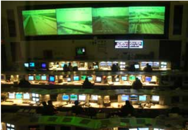
ITS Technology is typically monitored from a regional traffic control center such as this one in Houston, Texas.
