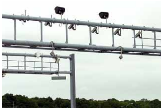
Electronic tolling technology has become standard on HOT networks.
